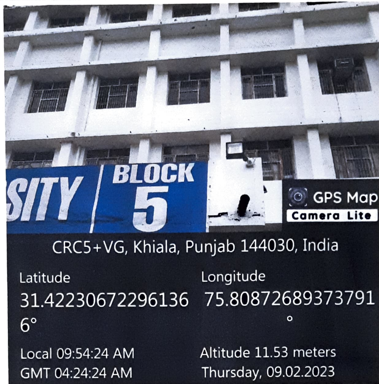
Figure: Lights installed in front of block 5
